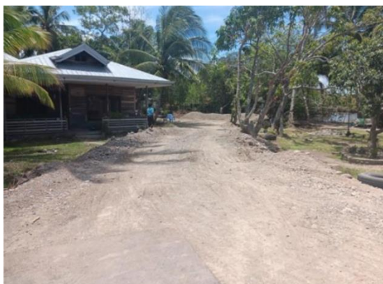
The dirt ramp that had to be built in order for the trucks and other heavy equipment to reach the pond
