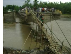
People trying to cross the collapsed bridge
